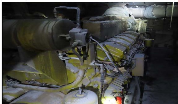
Figure 1: Damage sustained to auxiliary engine room
